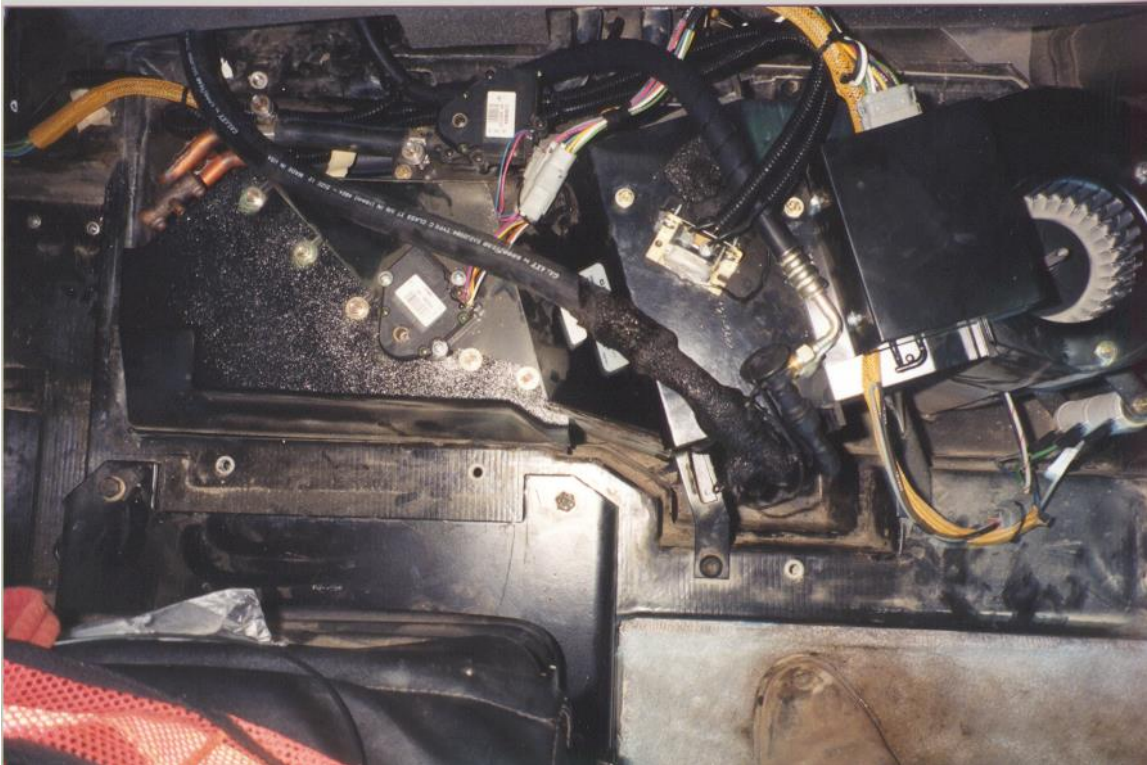
Evaporator box reassembled with hoses.
